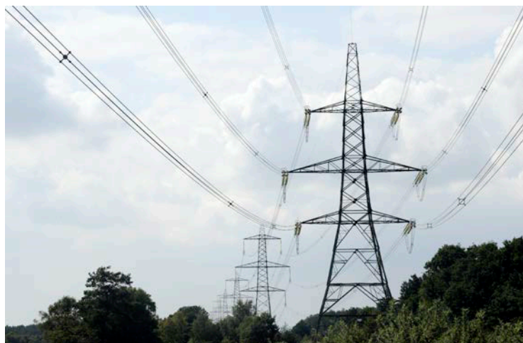
Figure 1 275 kV transmission line
