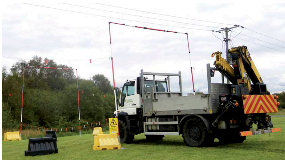
Figure 5 Typical passageway through barriers
