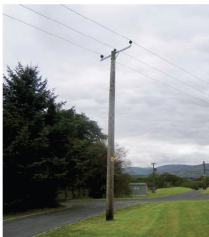
Figure 2 11 kV distribution line
